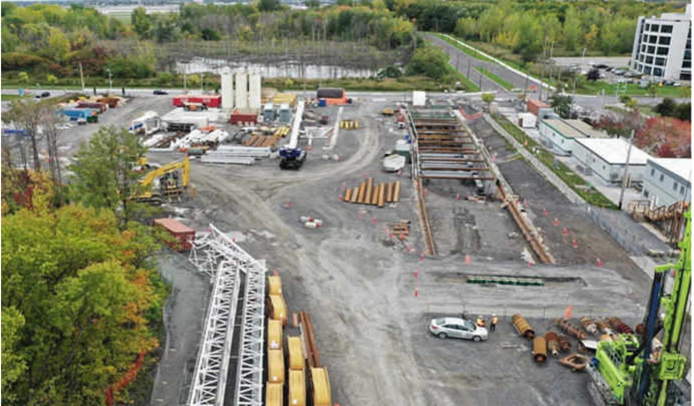
Destruction at the Technoparc Wetlands
